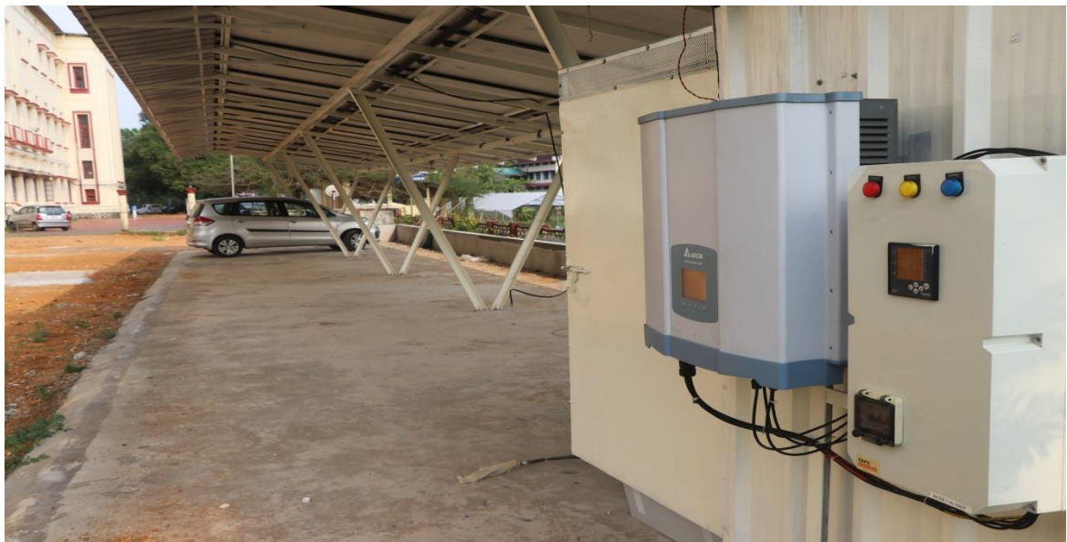
Solar Energy Harvesting Plant
